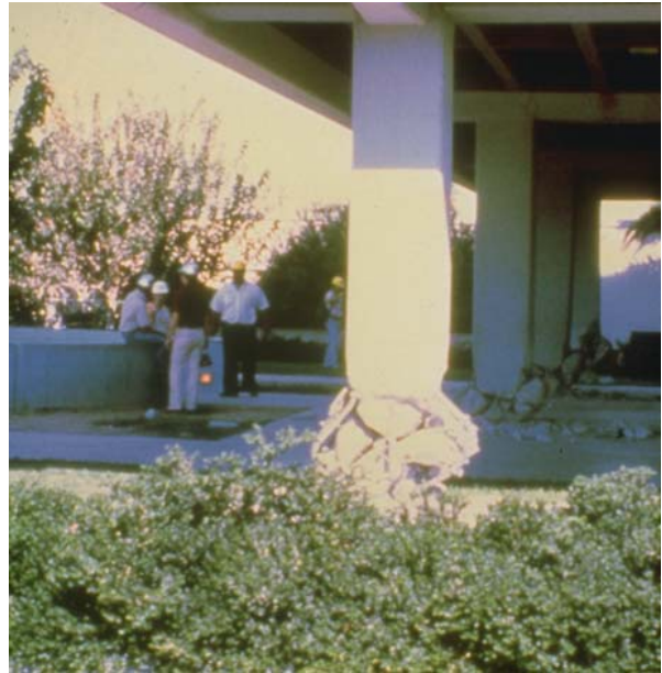
(b) Failure of columns at the base
